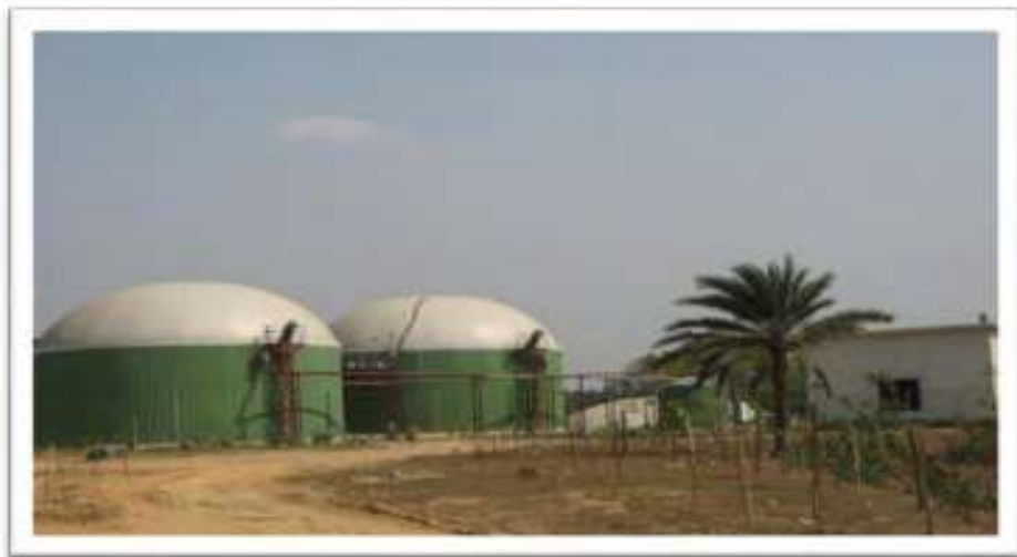
Biogas plant by Paragon Poultry Farm running a generator of size 206 kW
